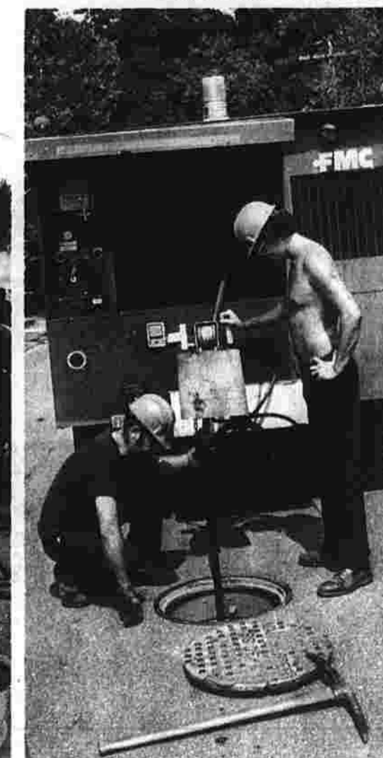
Cliff Carlson, left, and Dennis Armstrong inspect a sewer line on Marion Dr. The piece of equipment is a sewer jet, which cleans lines by air pressure. (Herald photo by Pearson)
